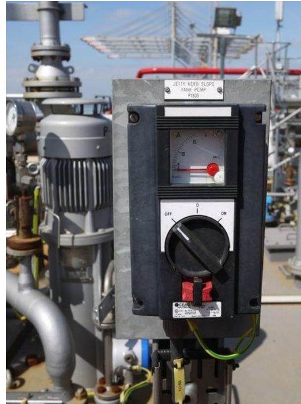
Pump start/stop. Design and layout consistent with others on site. Well located. No issues
